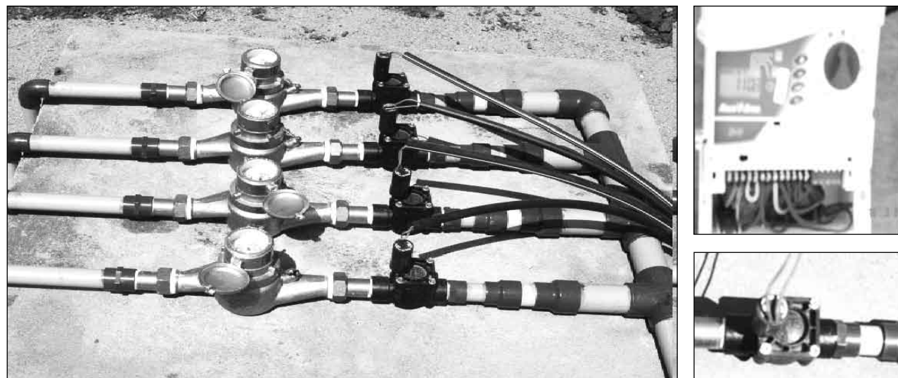
Fig. 1. The automatic drip irrigation scheduling hybrid stations controller (E-6) and solenoid valves
